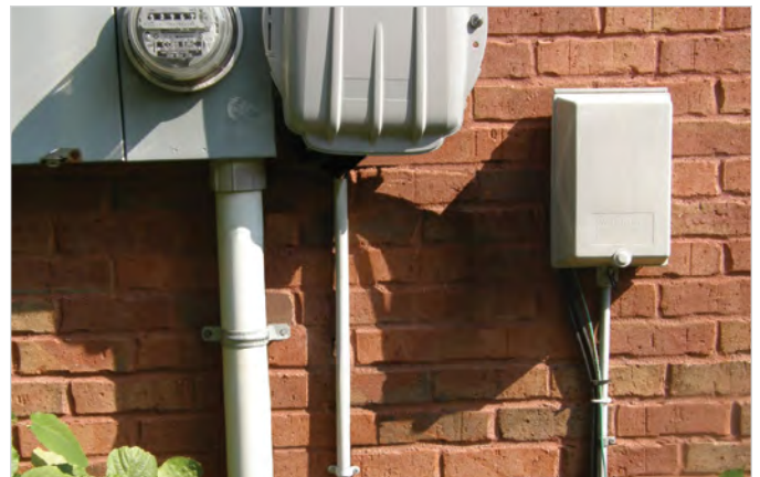
ONT closed with FTTP drop cable inside
