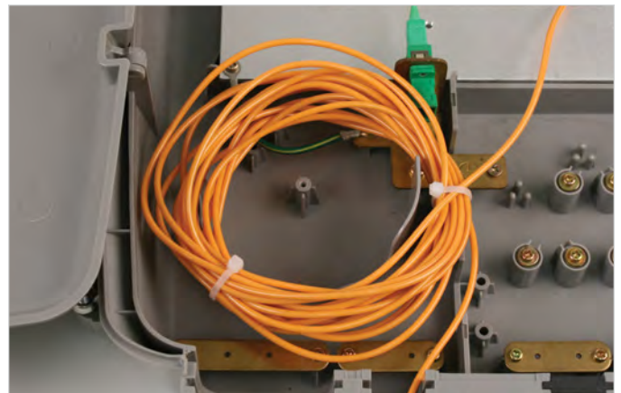
ONT open with drop cable secured and several feet of buffer tube coiled inside
