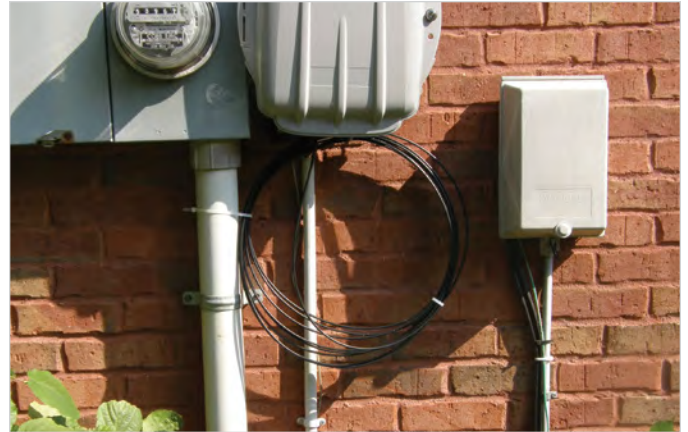
ONT closed with FTTP drop cable loop adjacent
