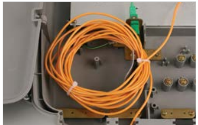
ONT open with drop cable secured and several feet of buffer tube coiled inside
