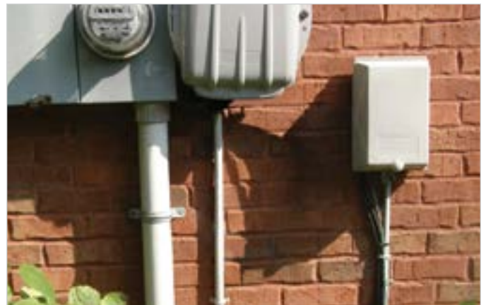
ONT closed with FTTP drop cable inside
