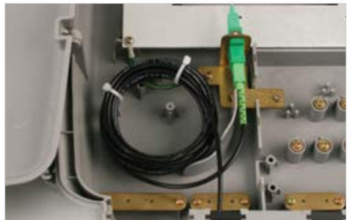
ONT open with W7 cable installed and tight coil of tight buffer drop shown.
